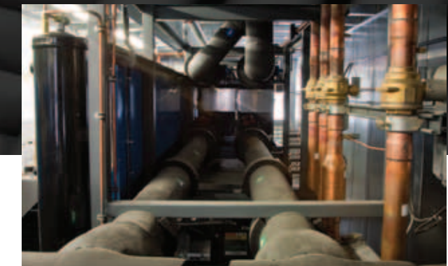
View of Dual Plate Chillers on SNMT Rack
