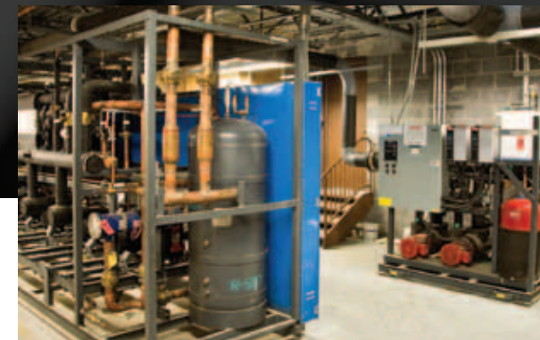
Installation of SNMT Rack (left) and SNPS with Variable Speed Control option (Right) in Mechanical Room
