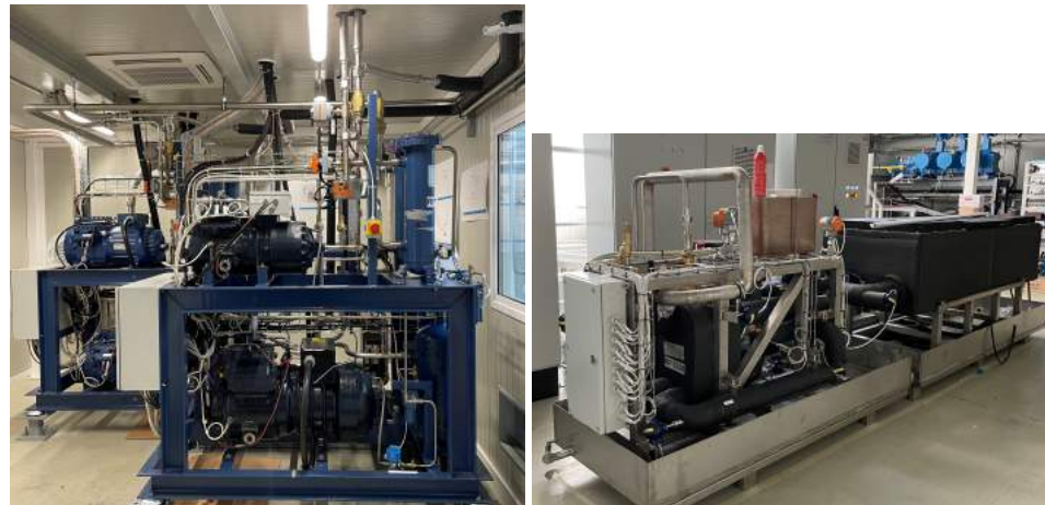
Figure 6. (left) Chiller room with two compressor slices and connections to gas coolers and common unit (right) Dummy load used to replicate operation of 2PACL system and heat load.
