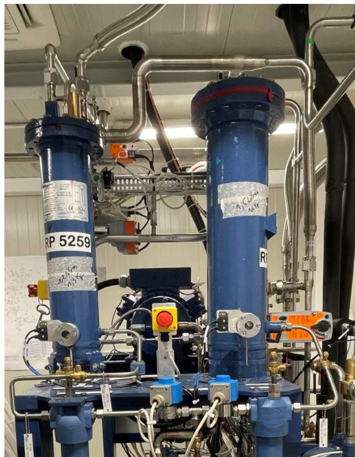
Figure 7. Coarse and fine oil separators installed in one of the compressor slices.
